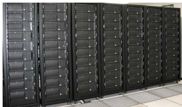
Figure 4. Large Commercial Installation
