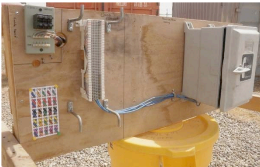
Figure 4. We built a mockup telephone punch board for hands-on infrastructure training.
